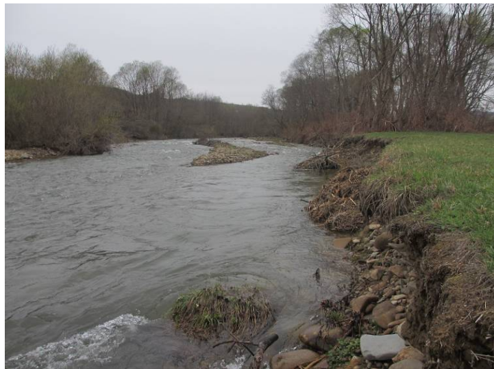
Fig. 12. Suci River left bank erosion at 9\text{m}^3/\text{s}
